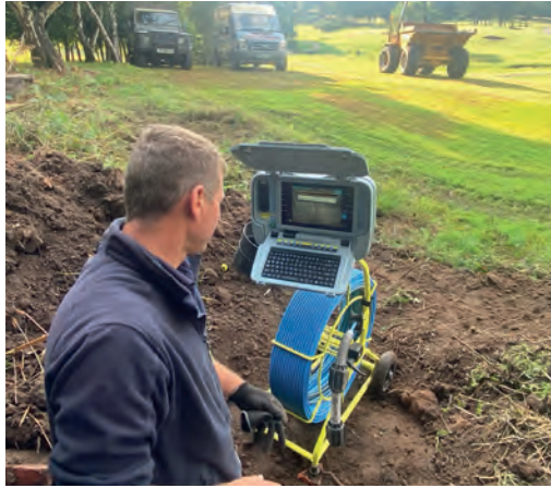
Below Philip Dixon Contractors with drainage camera inspecting existing drainage for any issues.
