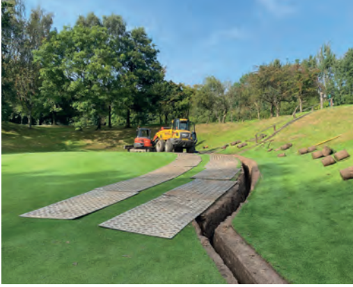
Left Drainage installation around the 2nd green, part of the annual drainage investment plan.
