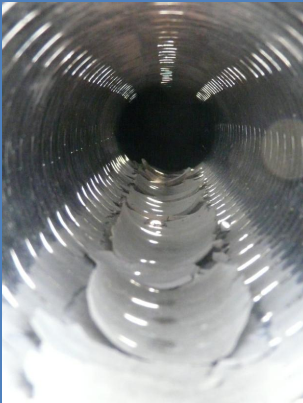
Silt from liquefaction deposited in a lateral pipe drain at the AMI Stadium.
