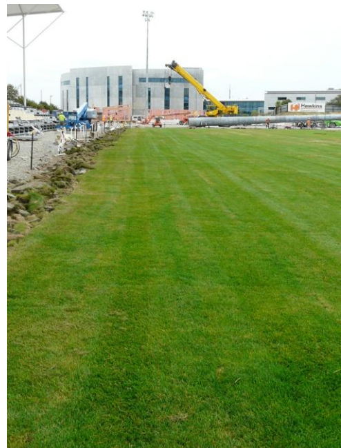
Turf first laid on 7/2/12 already knitting in. The lighting tower awaiting installation in the background has been recycled from Carisbrook. One of the new stands can just be seen to the left of the photo.
