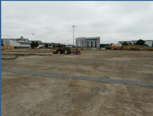
Levelling, lateral drainage and irrigation work at the Christchurch Temporary Stadium, Addington (January 2012).
